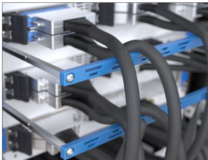
Rack Utilizing Cable Support Management Kits
