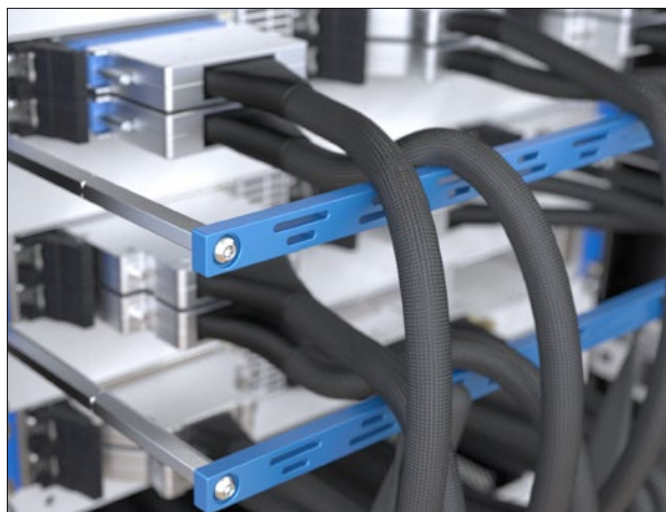
Rack Utilizing Cable Support Management Kits
